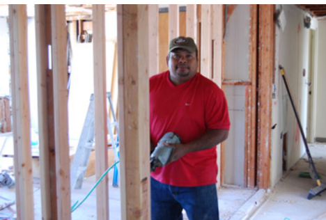
Jaime Flores, framing carpenter, is roughing in the new data room, 3rd floor.
