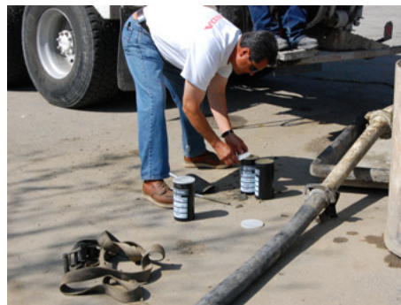
Deputy Inspector Jose Sigala takes samples of the concrete to check the slump and mixture of the concrete.
