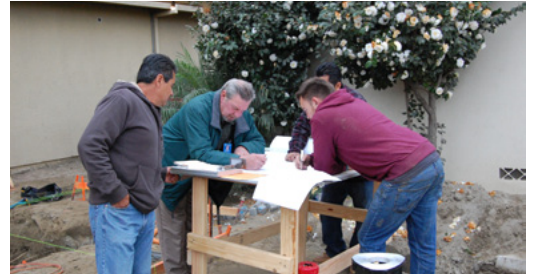
Building Inspector Kris Anderson, City of Bellflower discusses with Deputy Inspector Jose Sigala, Alex DeLeon, Vincor and Alfredo Urbina, Project Supervisor about the dowel sizing for the steel cage.
