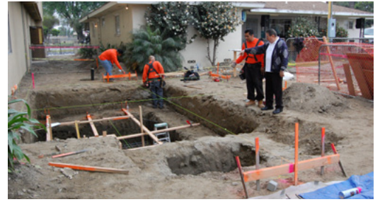
Fr. Joe Farias speaks with Alfredo Urbina, Job Supervisor, Vincor about the elevator pit construction.
